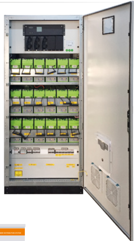
110VDC/200A, Hotswappable/Upgradable DC System in IP41 Cabinet with 2 Groups of 12V FT Batteries and Remote Access
